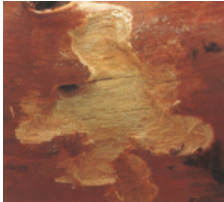
Roundheaded borer tunnel
